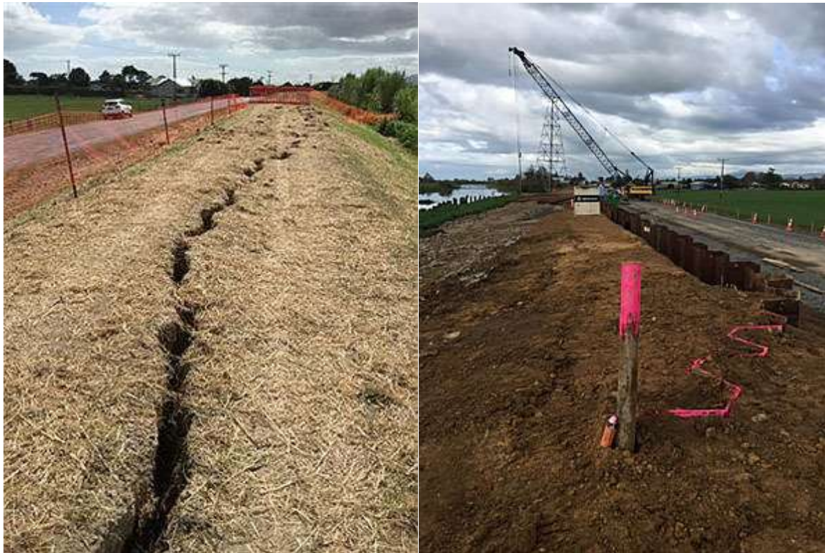
A major issue is that the deep marine mud soils have limited load carrying capacity, leading to stop-bank stability issues as shown above near Ngatea. More expensive sheet piles provide a solution
