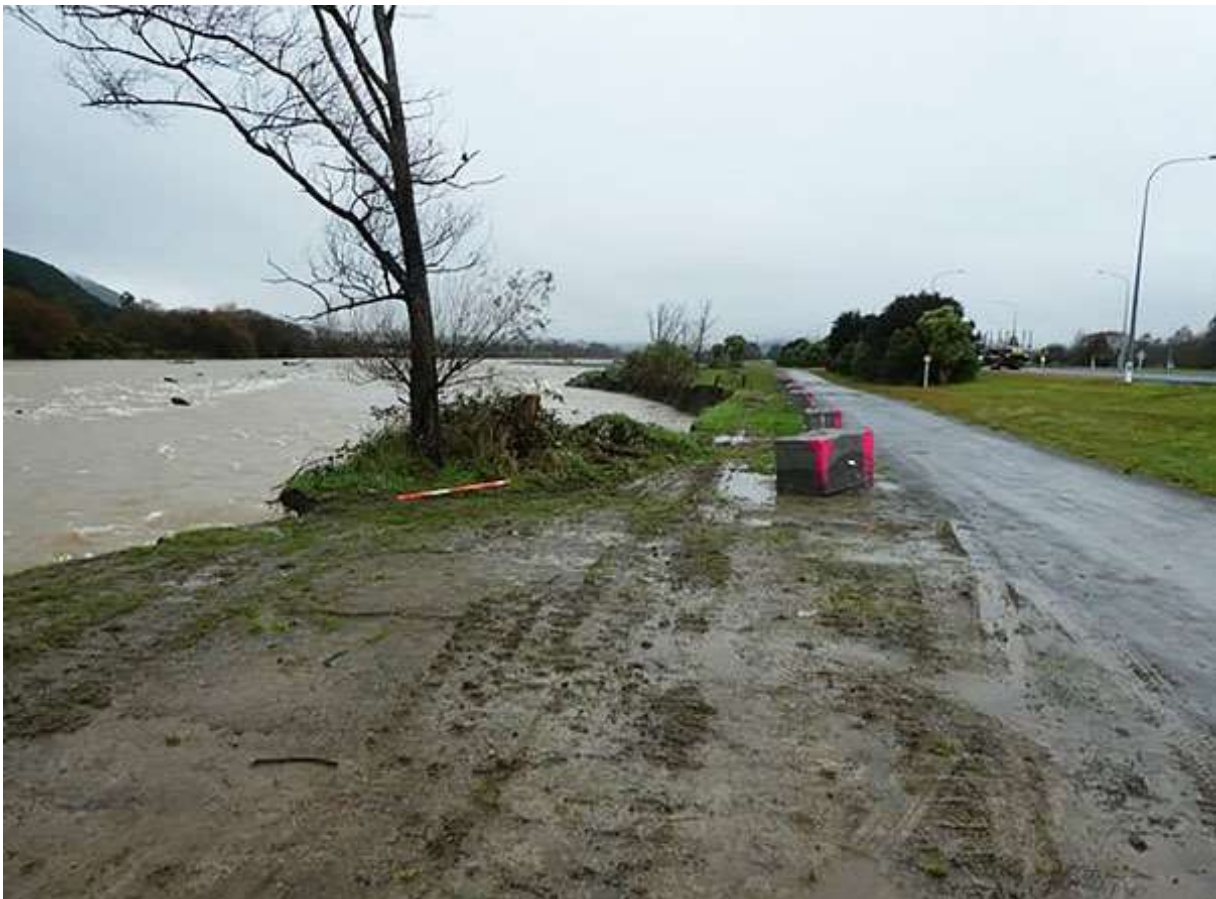
Hutt River erosion adjacent to State Highway two during a small annual flood event in June 2018
