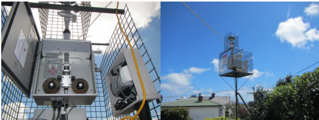
Figure 2: The original E-BAM monitoring system set-up and installation at Central School, New Plymouth. This equipment was upgraded in July 2022.
