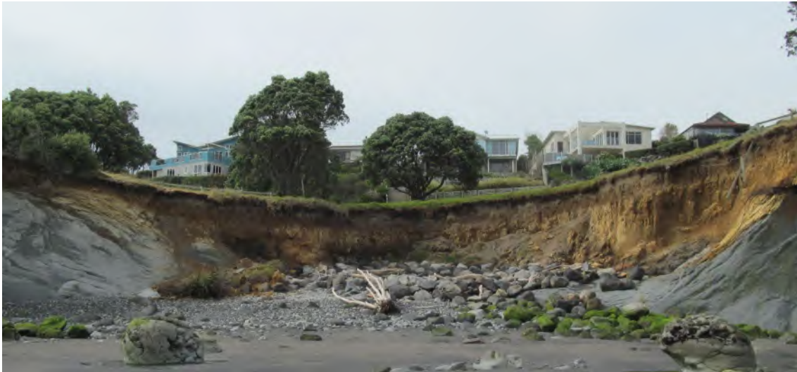
Coastal Erosion at Motukari Reserve, Onaero
