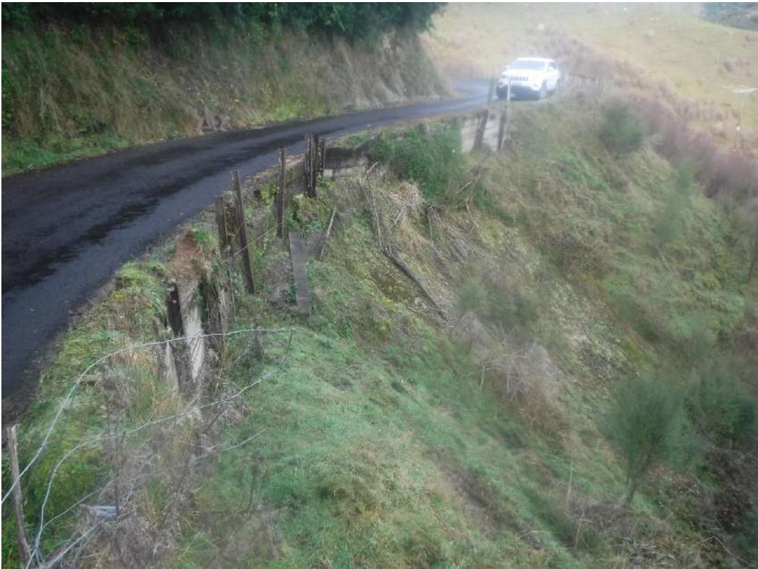
Figure 5 – Mohakau Road Retaining Wall at RP3380 to be replaced
