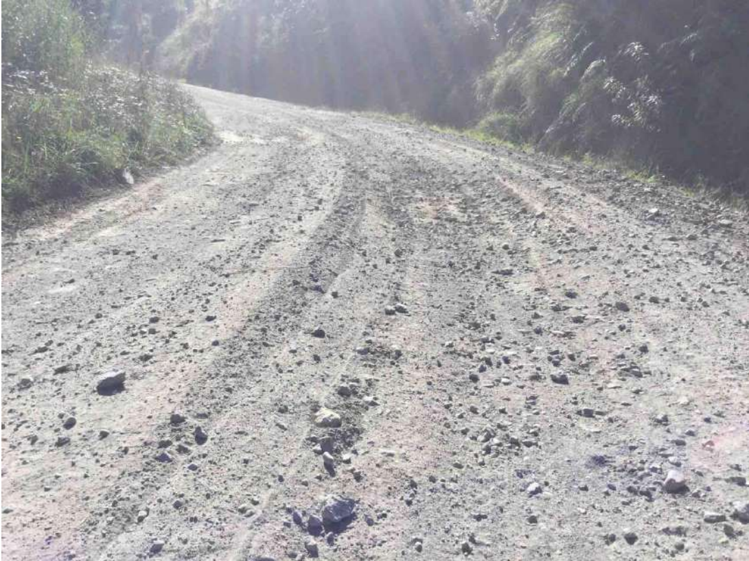
Figure 1 – Pavement damage to Puniwhakau Rd
