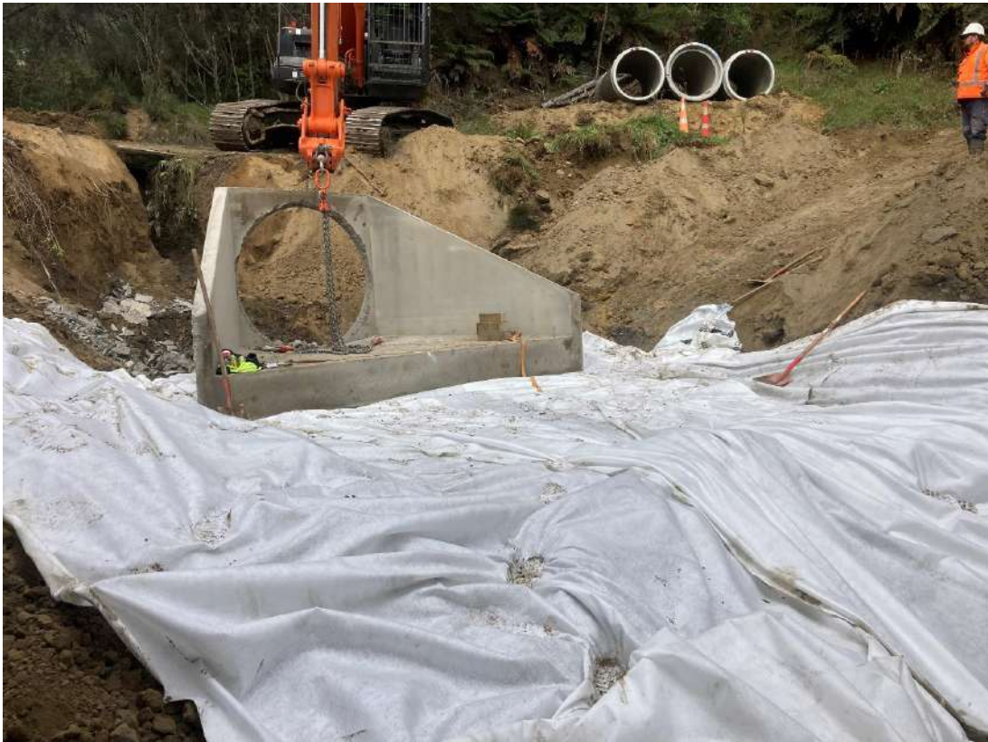
Figure 7 – Installation of the wing wall at the outlet of the new culvert. Note the existing water drive in the background.
