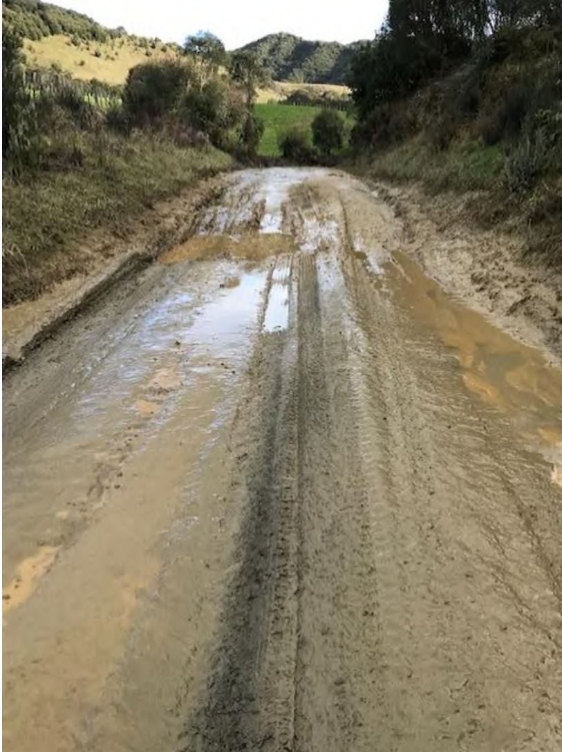
Figure 1 – Pavement damage to Puniwhakau Rd
