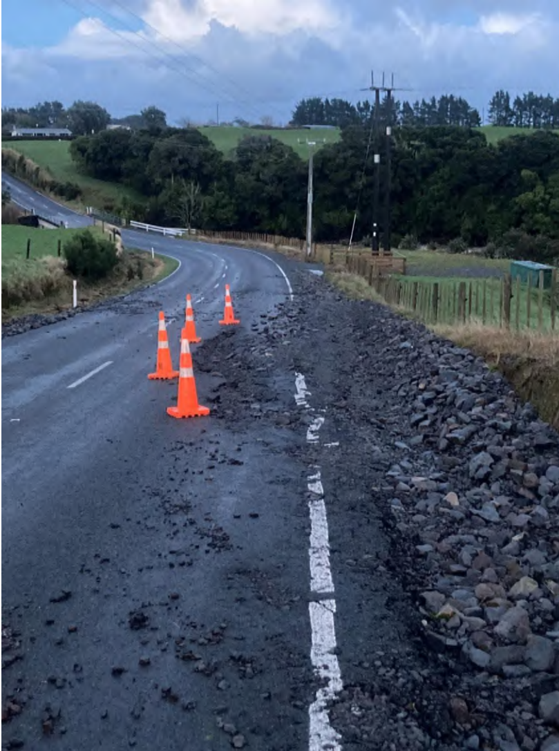
Figure 3 - Extreme rainfall event causing damage to Palmer Road.
