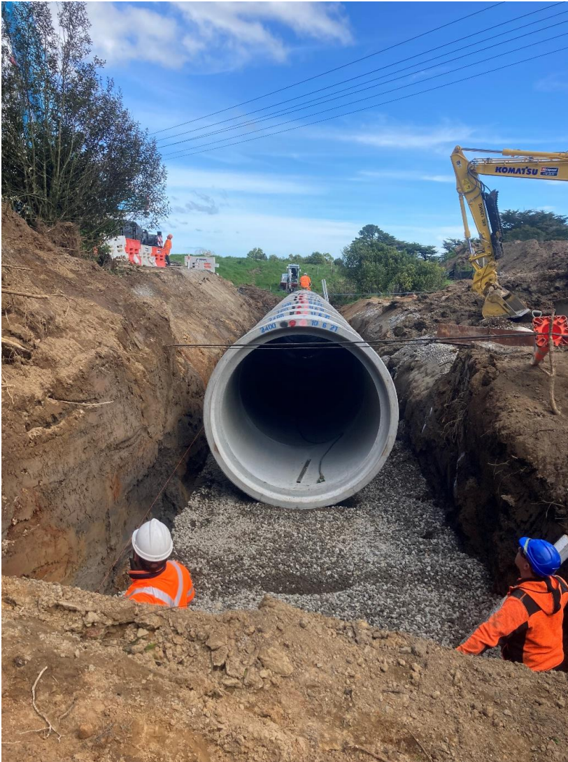
Figure 6 – The replacement culvert on Manaia Rd at Hollard Gardens. Note the size of the culvert is due to meeting the New Environmental Standards for Freshwater.
