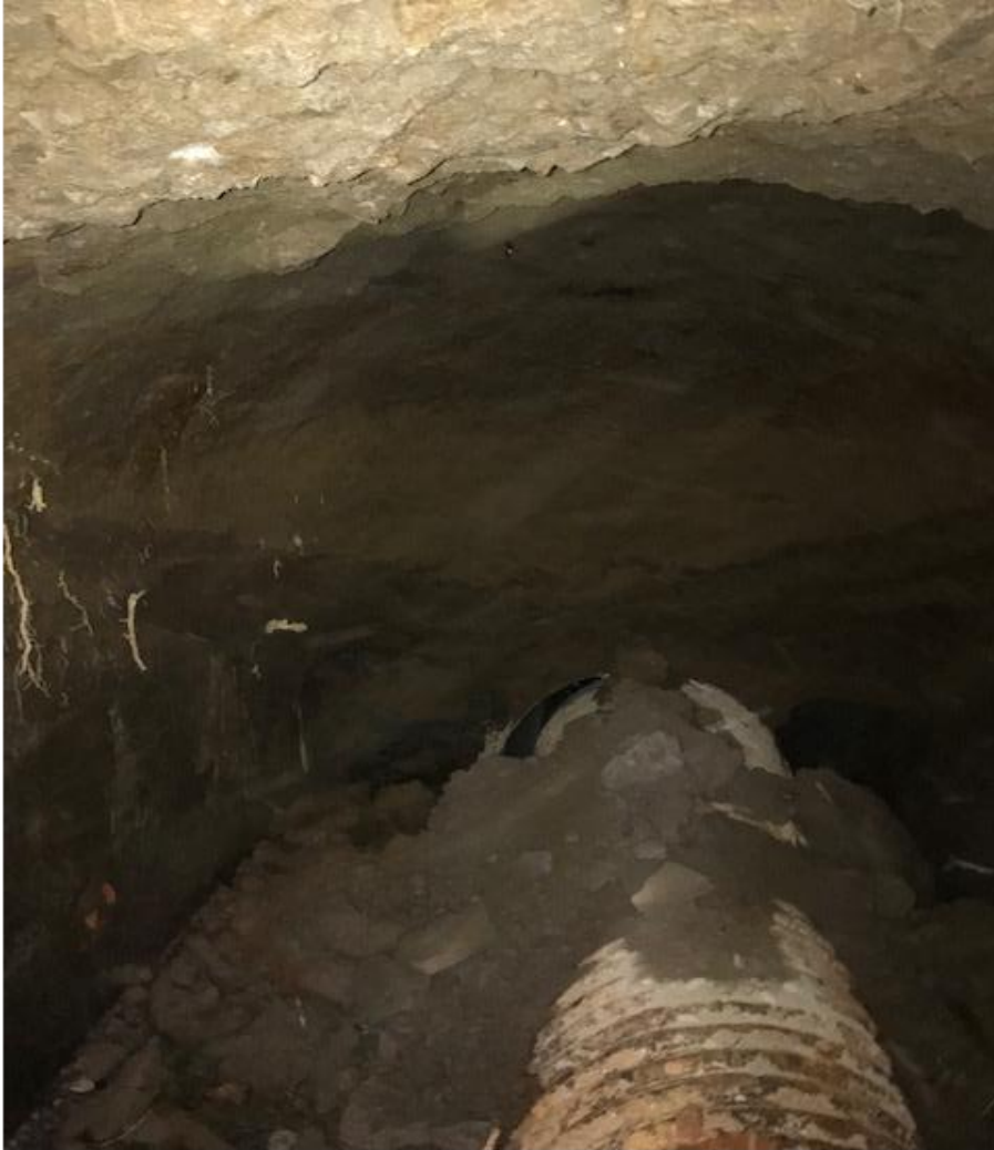
Figure 4 – Collapsed culvert under Manaia Road. This cavity is approximately 6m long x 1.5m high and 3m wide. Note the gap between the two culvert pipes at the joint
