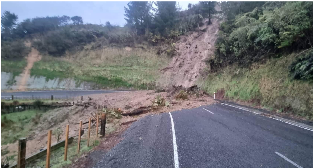
Figure 3 – Slip blocking Mangaotuku Road
