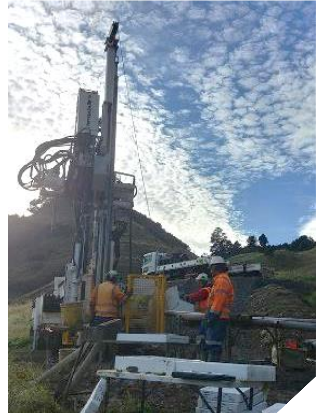
The crew at Te Oreore site drilling boreholes and installing groundwater monitoring devices, deep within the landslide area
