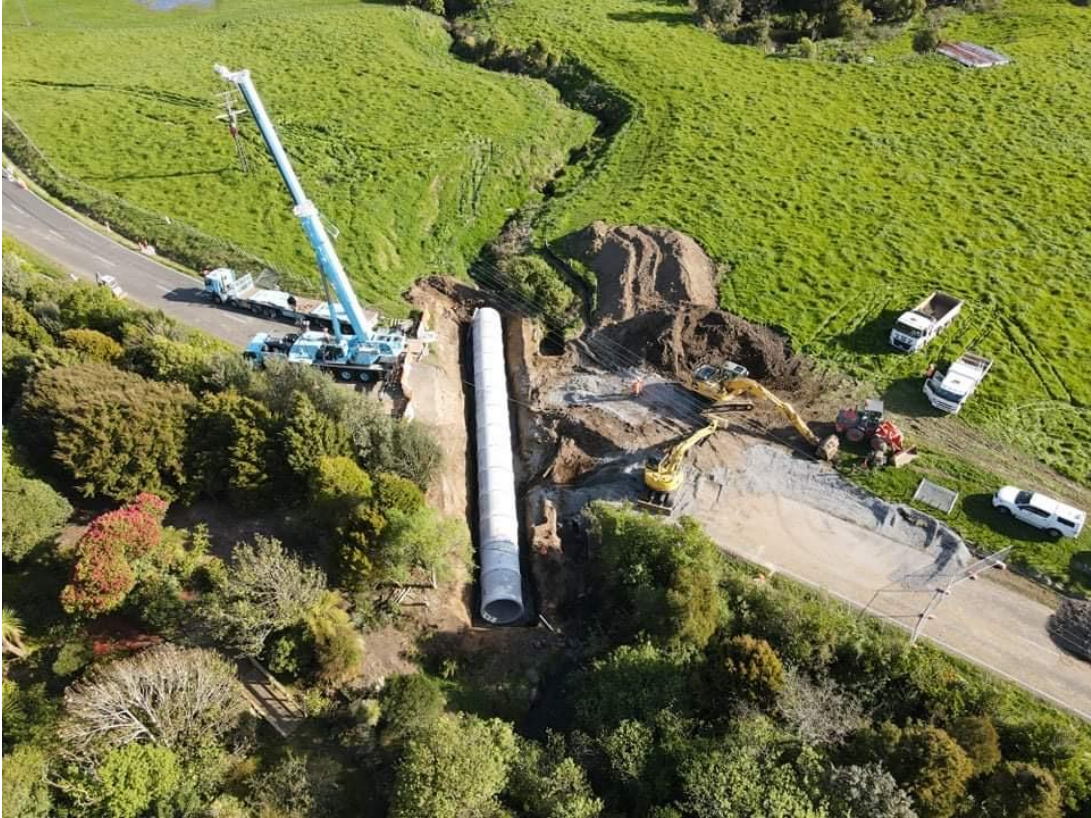
Figure 7 – Aerial photograph of the new culvert installed on a new alignment alongside the existing steel culvert.
