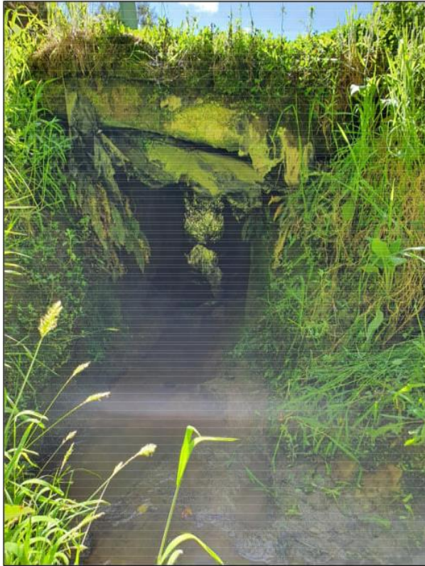
Photo 1: Inlet to the water drive
