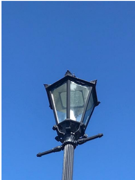
Streetlight in Mercade Close.
