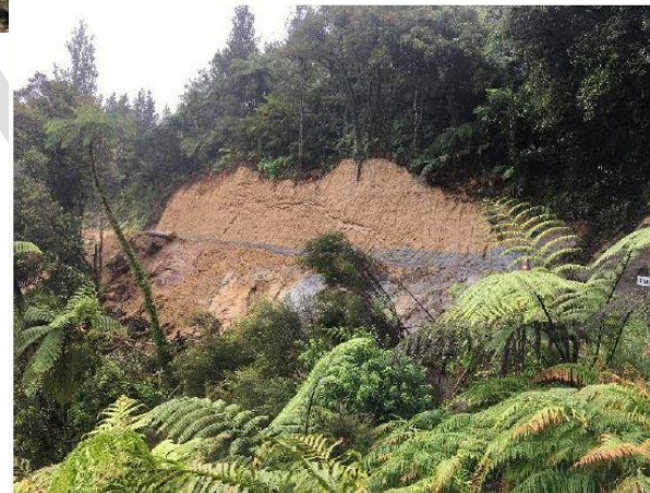
Safety Improvement on Junction Road where a logging truck rolled over down the bank on a narrow section of the road.
