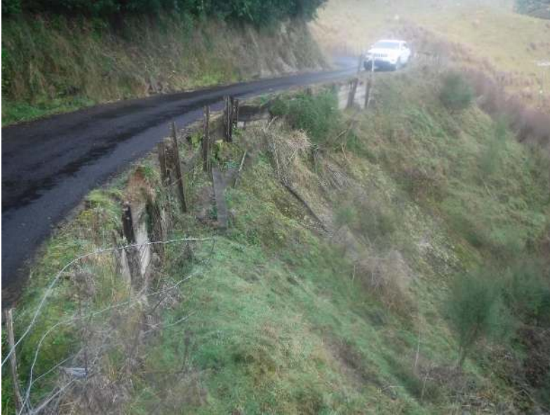
Figure 4 – Mohakau Road Retaining Wall at RP3380 to be replaced
