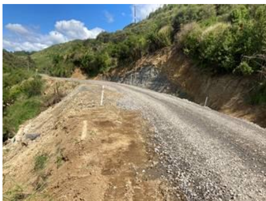
Figure 3 – Bank retreat on Mangare Road.
