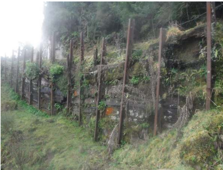
Figure 5 – Retaining Wall on Mohakau Rd at RP3430. Horizontal boards to be replaced.
