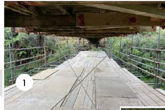
1. The finished underside before removal of the scaffold and final tensioning of the hand rails
