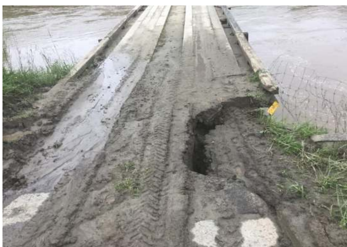
Figure 1 - Damage to the land span of McBride's Bridge.
