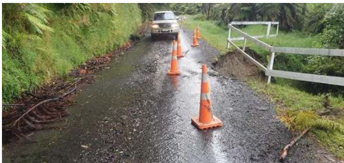
Figure 2 - Underslip on Mangaoapa Rd north of the Matau Tunnel
