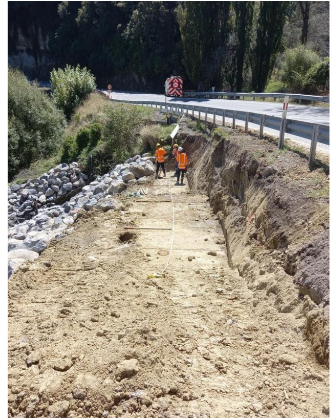
The crew in March at the prepared base for the gabion retaining wall at the Southern End roadside.
