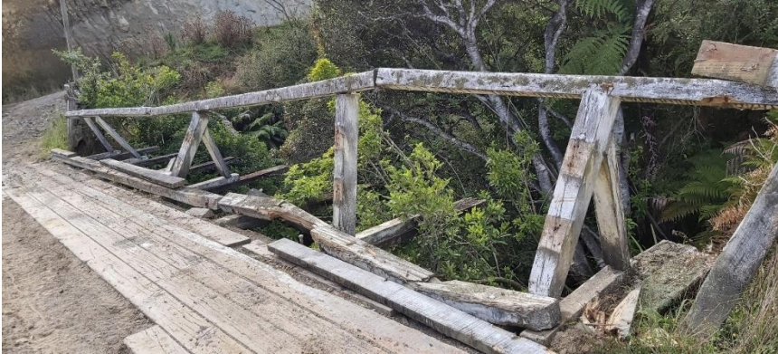
Figure 2 – This damage was caused by a logging contractor on 16 March 2022.
