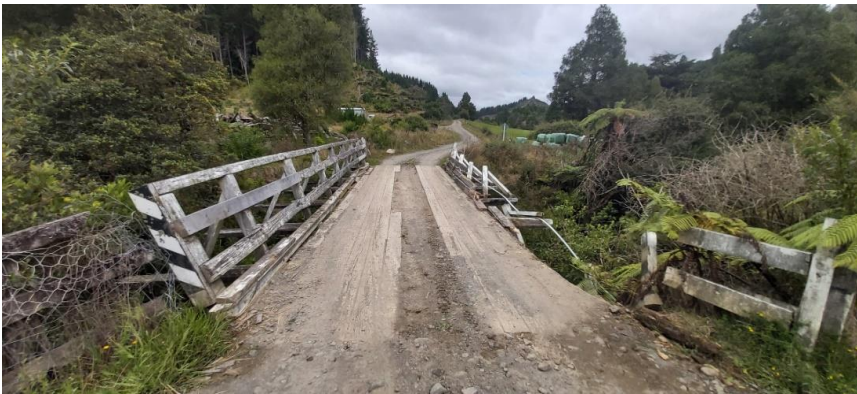
Figure 1 – This damaged was caused by a logging truck on 22 February 2022.
