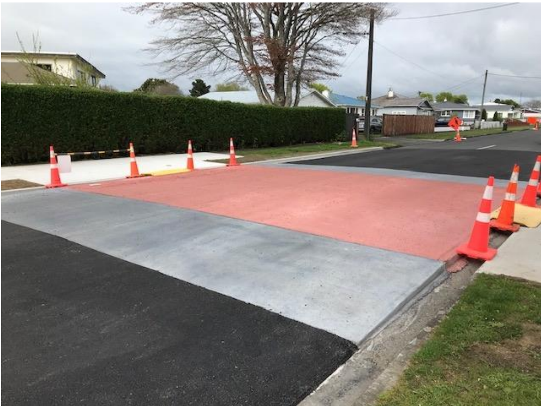
Figure 8 – Stratford High School Safety Project – Works in Progress showing the new raised platform at Cloten Road.
