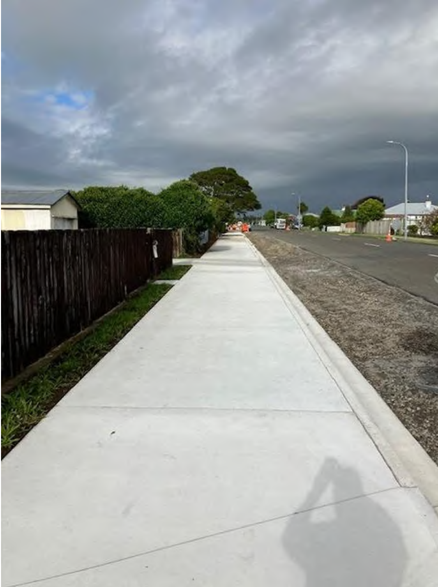
Figure 8 – Replacement of the footpath on Fenton St to provide a shared use walkway/cycleway.
