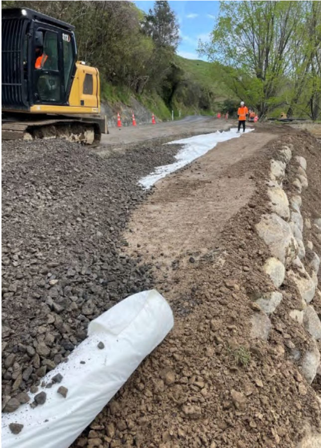
Paparata Hill dropout repair
