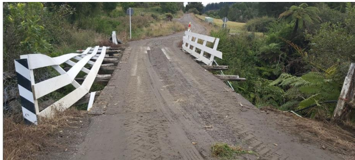
Figure 5: Damage to the bridge located at the end of Puniwhakau Rd.
