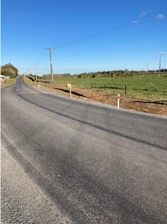
Figure 5: Work to re-shape the 45km/h corner known as “Hick’s Corner” on Beaconsfield Road.
