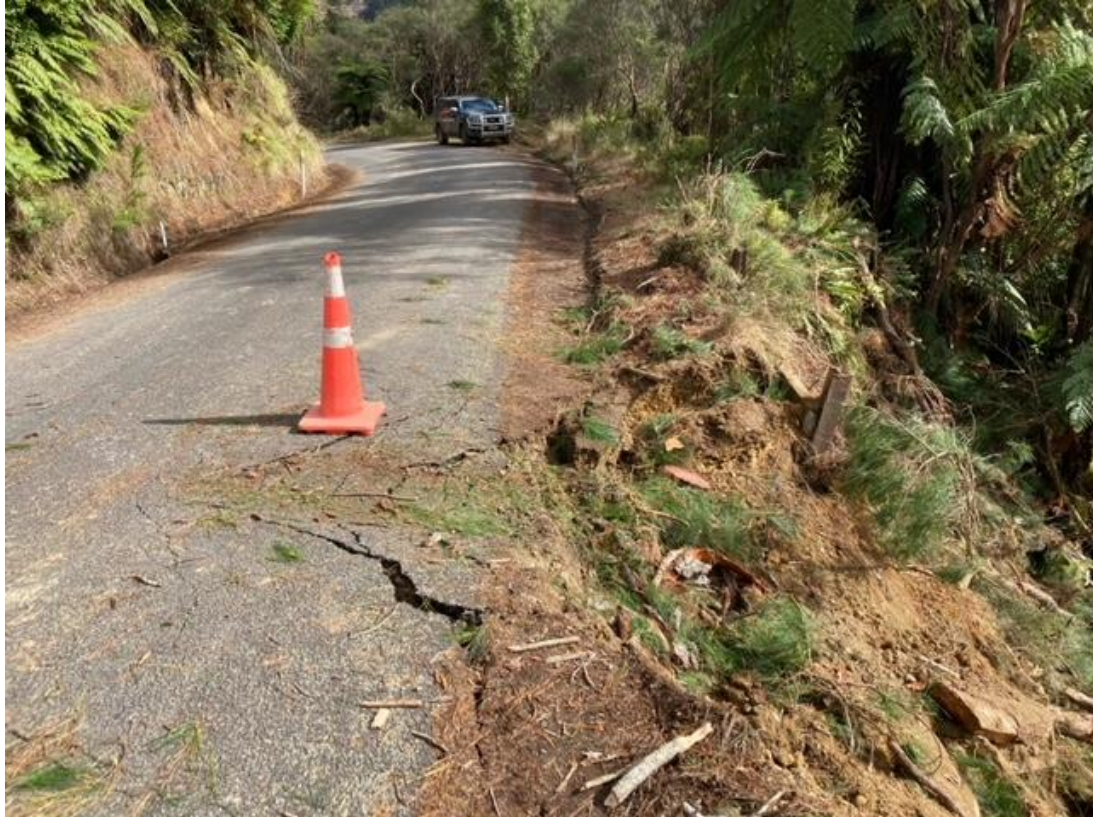
Figure 10: Damage to a retaining wall and road surface on Matau Road.
