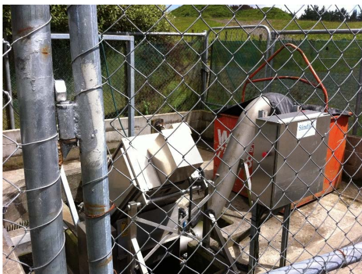
FIGURE 3: Influent Step Screen, Screw Conveyor and Sealed Bin
