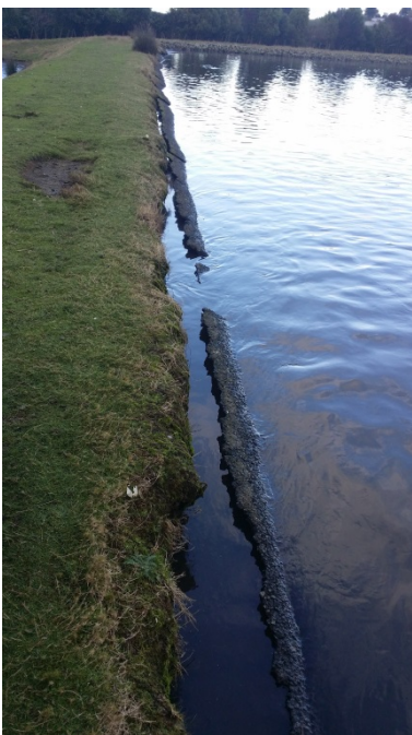
Photo 3 Waveband erosion June 2015
