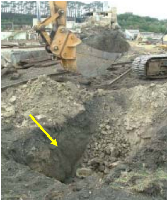
Pit 7 (825) 2637370-6159394 Under rail line, blackened gravel to 0.4m then natural ground, sampled dark material at 0.3-0.4m
