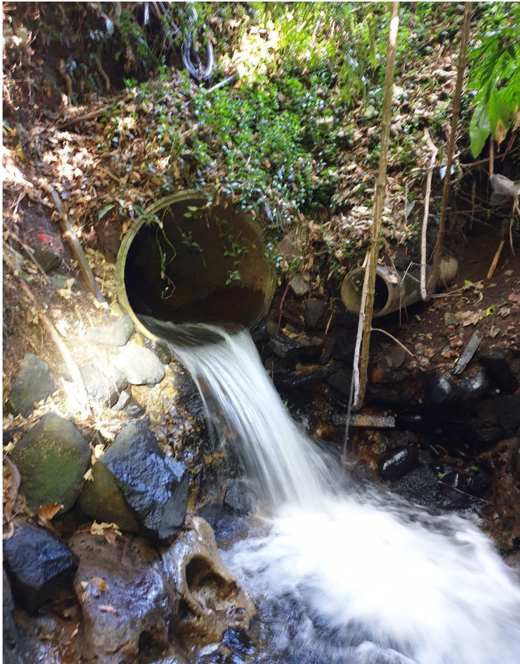
Photo 2 Culverts like this one create a barrier to fish passage.
