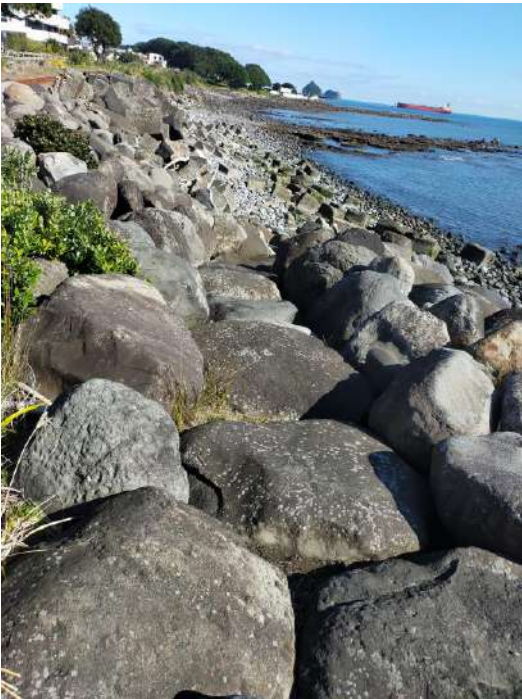
Figure 35 – Photograph showing example of rocks placed in revetment to allow for informal public access down revetment.
